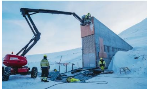
Construction workers add the finishing touches to the seed vault. Photograph: Ragnhild Utne/Statsbygg
